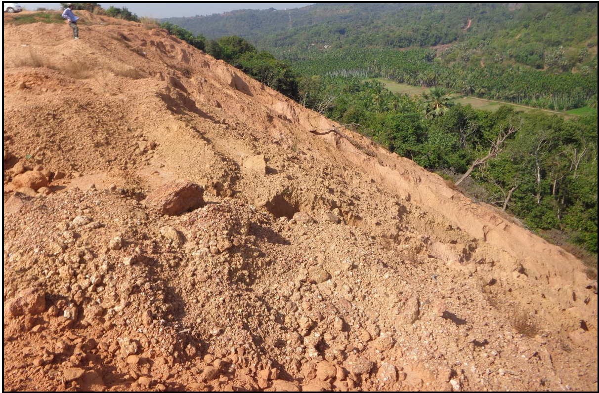
Photo 15: Loose debris hump on the downslope side along the road, North of Farangipet
