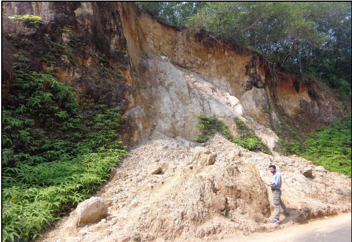
Photo 24: Debris slide initiated by road cut ,triggered by rainfall along the Kollatadaka-Delantamajalu road
