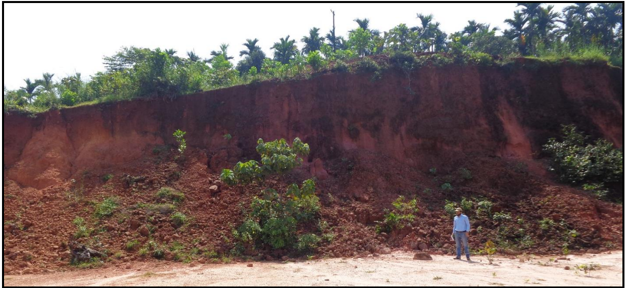
Photo 1: Extensive cut slope in soil near Punjalkatte
