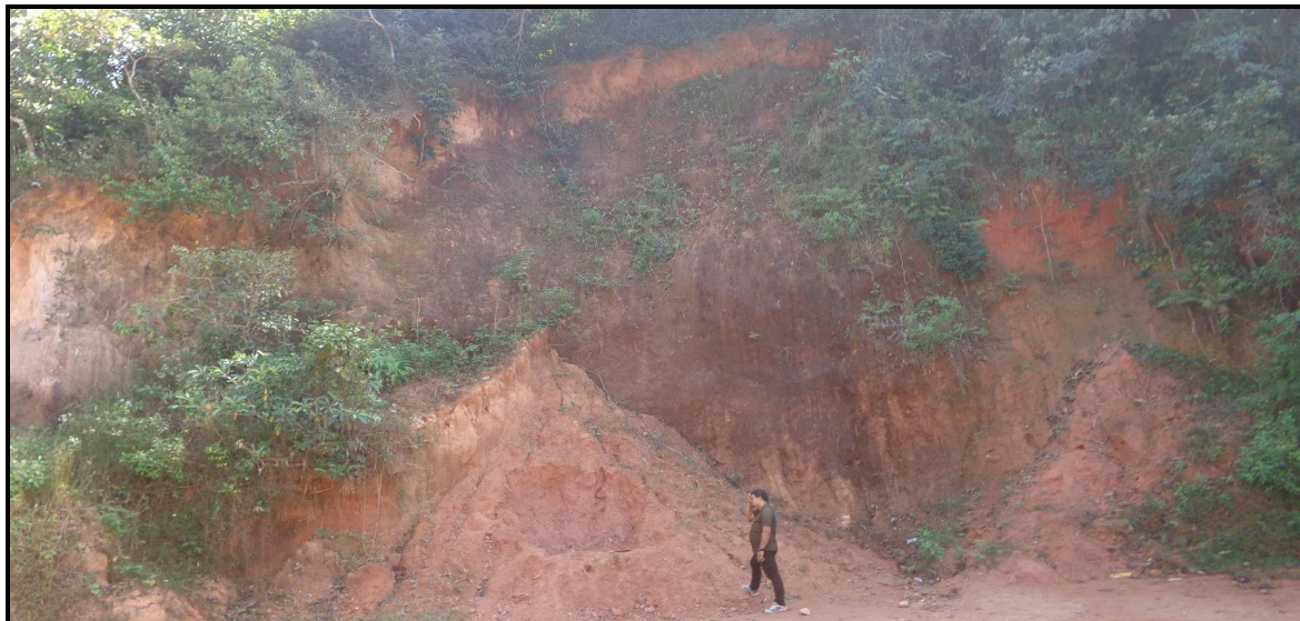
Photo 25: Debris slide along the road section Kabelá-NH-48
